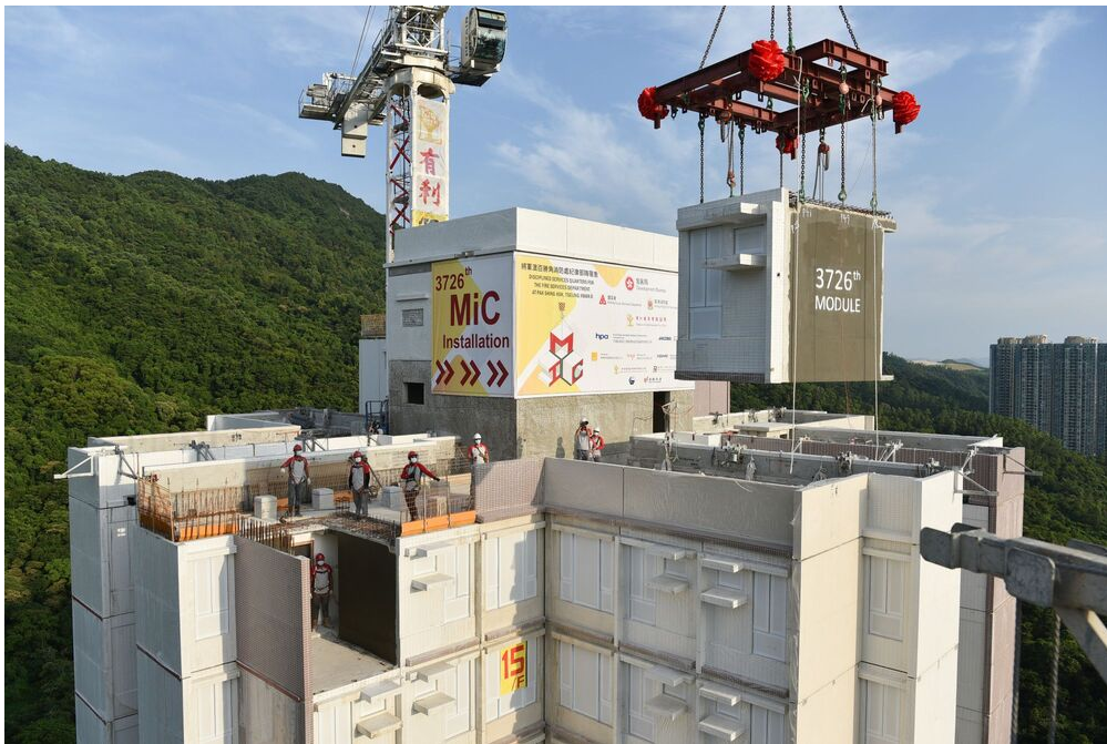
Figure 3: On-site crane assembly of MiC modules for a residential building, illustrating the stacking process that replaces conventional floor-by-floor construction. Source: The Standard, https://www.thestandard.com.hk/news/article/186351/
