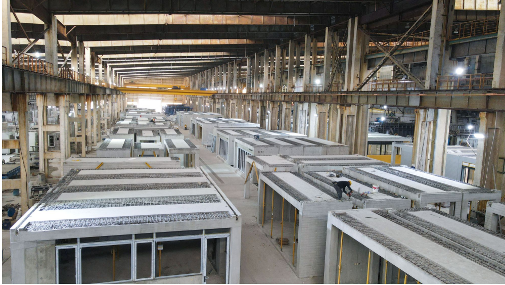
Figure 2: Factory production line for MiC modules, showing completed bathroom and kitchen units being assembled under controlled conditions before delivery to site. Source: Development Bureau, HKSAR, https://www.devb.gov.hk/filemanager/en/content_1044/20240414_02.html
